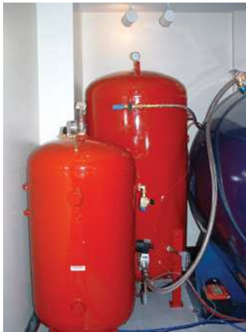
Deluge + Hand-line Fire Suppression System Included
